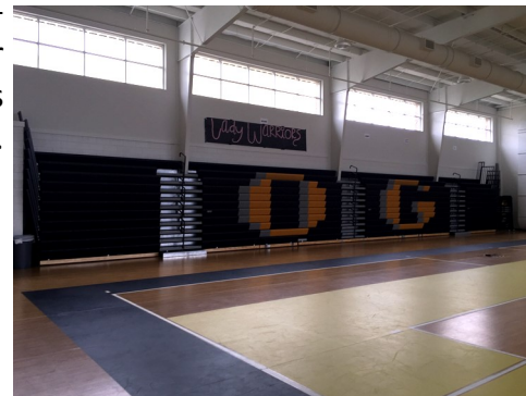
Installation of a Universal seat module system at Oak Grove High School Volleyball Gym.
